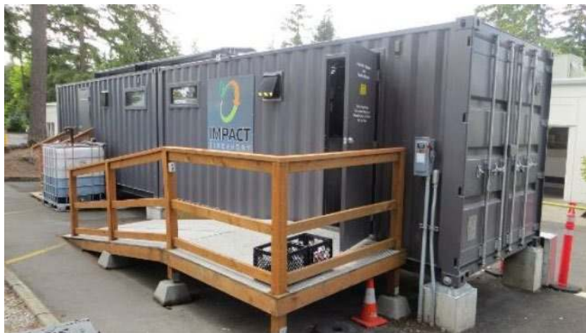
Figure 3.2. Impact Bioenergy modular anaerobic digestion system.
